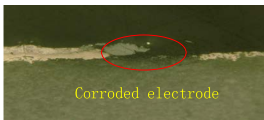
Figure 1 Left top terminal is corroded
